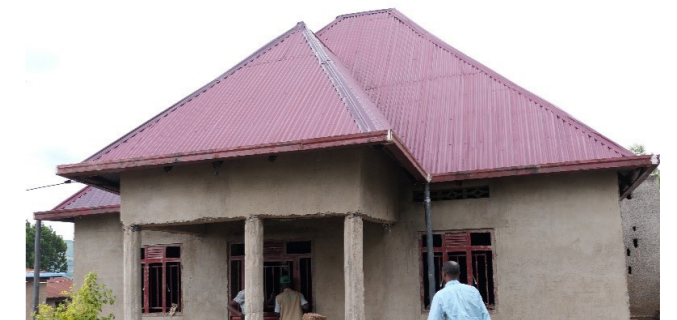
Jean de Dieu is constructing a modern house which will be completed in June 2024.
